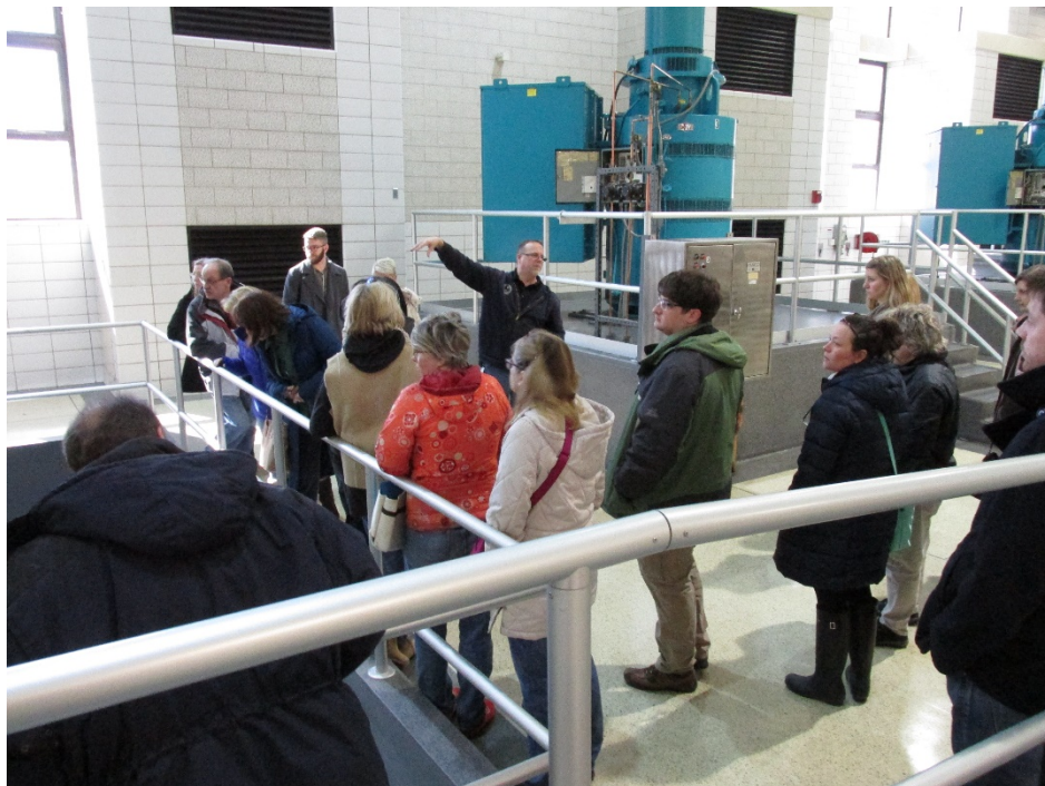
Mike Weed pointing out the pumps below
